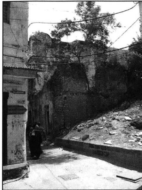
Picture 8: Crumbling building stock
