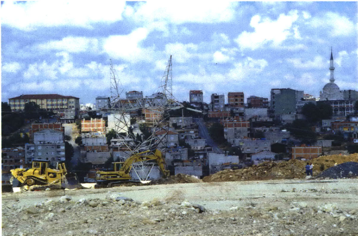
11. Bulldozers working at the edge of the Olympic stadium parking lot, with a residential neighborhood seen in the background
