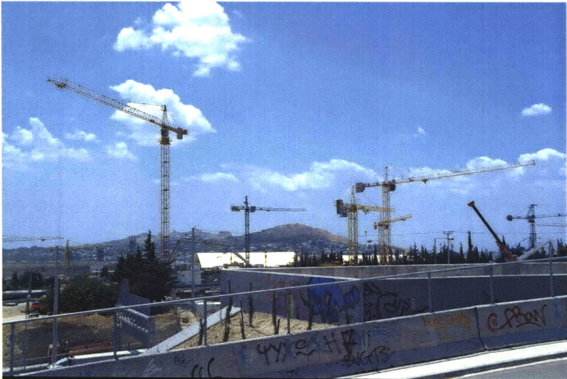
7. View of cranes at work at the Athens Olympic Sports Complex (OACA) to the north of the city as seen behind a fence and concrete blocks along a new highway intersection
