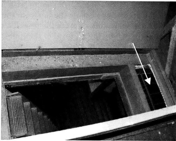
Figure 4-14 Pre-existing aperture adjacent to pull-down stairs. The large opening at left was not available for airflow since the Attic stairs were closed except for infrequent trips to the Attic for maintenance or storage. Shown at right (white arrow) is the small, fixed aperture that was previously kept unobstructed throughout the summer season. At the top of the photo is an insulated exterior door that swings down to seal all the openings in the winter season.
