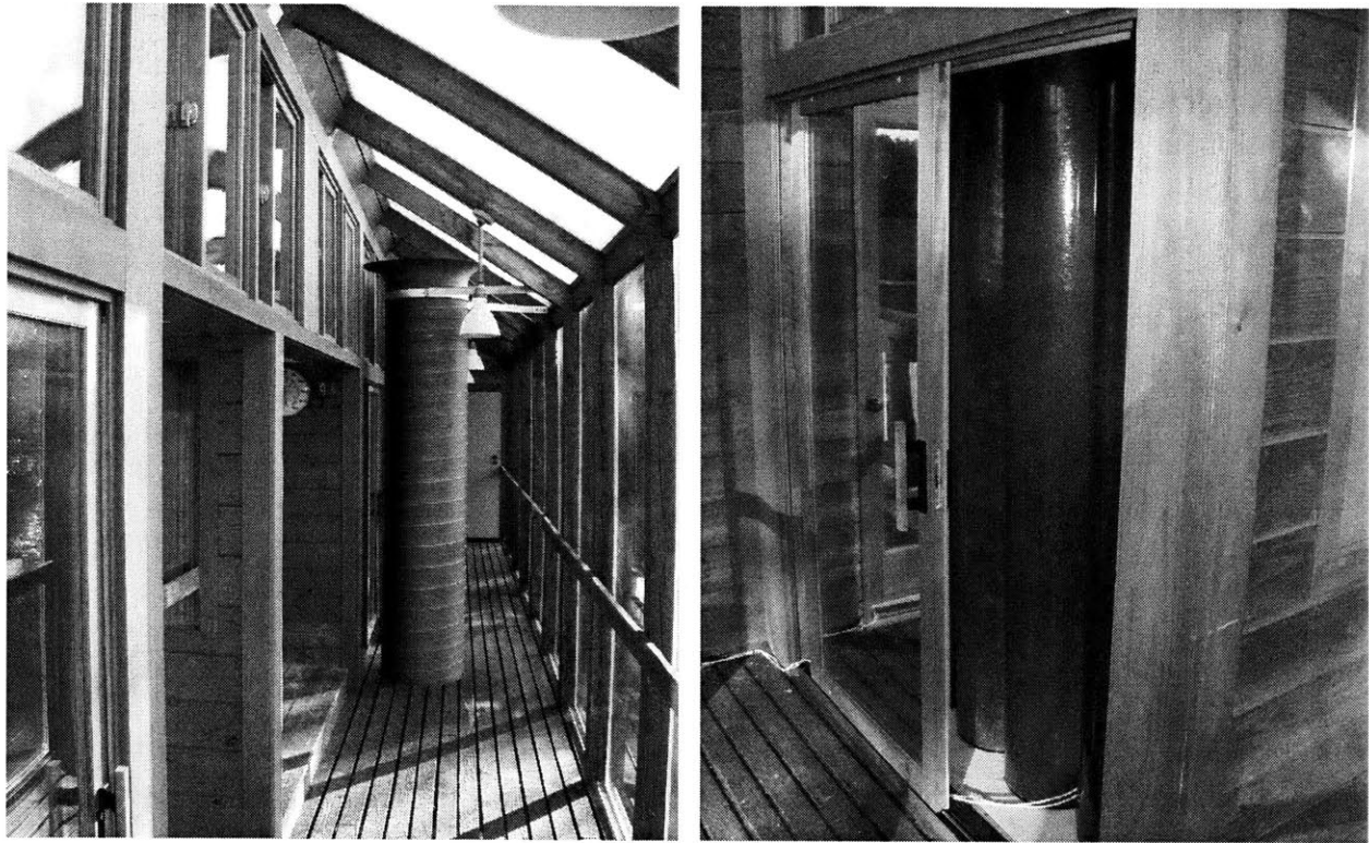
Figure 4-12 Upper level of Sunspace. Slats in the floor (1/2") permit some exchange of air with the lower level of the Sunspace. Left : View towards East. In the Fall and Winter, a fan moves hot air from the top of the Sunspace through the duct in the center of the photo to the rockbed below the Basement. The water wall is on the left side of the photo. The closed door at the East end of the Sunspace was open throughout most of the monitoring period to allow escape of hot air. Right : Detail of water wall, with slider open to show water-filled tubes.
