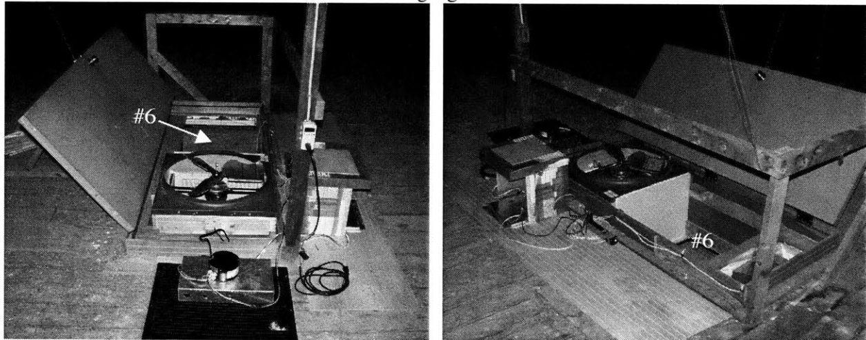
Figure 4-20 Installation of ECM-driven fan. Left: In the foreground, note the black motor controller on an improvised heat sink. This element was not in the airflow path and became very hot.
