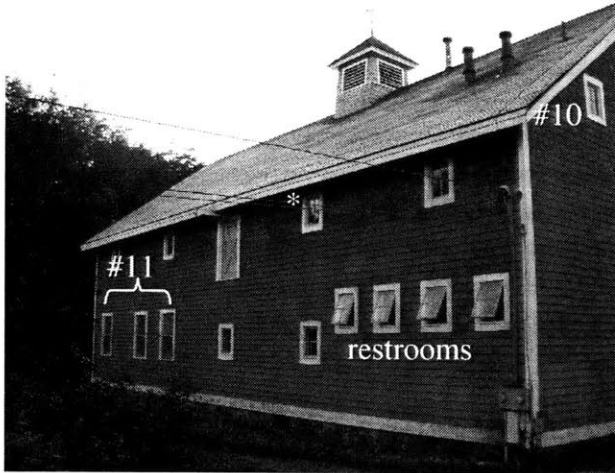
Figure 4-5 North face of building. Open windows at right are to vent the restrooms. These apertures were not carefully monitored since the restrooms are somewhat isolated from the rest of the building. The white asterisk (*) indicates the Attic 1 window above which the outside temperature thermocouple (thermocouple 10) was placed. It was placed under the eaves, protected from direct sunlight.
