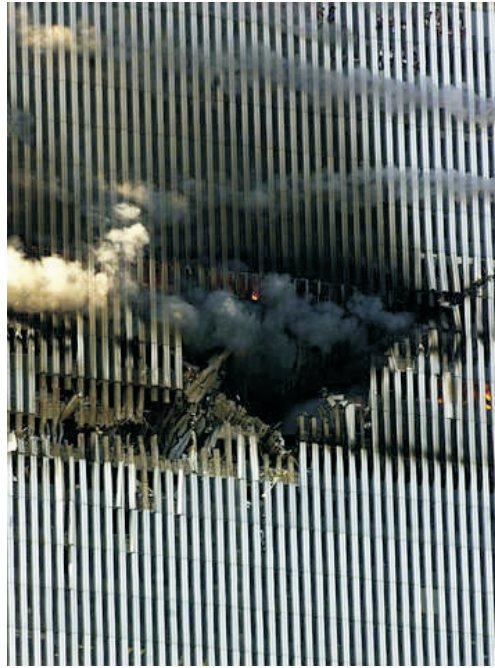
Fig. 1-1: A “clean” cut driven by the wings of a Boeing 767 into the facade of the North Tower [1].
