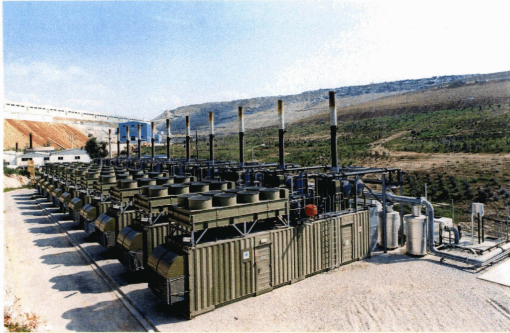
Figure 6: Natural gas plant
