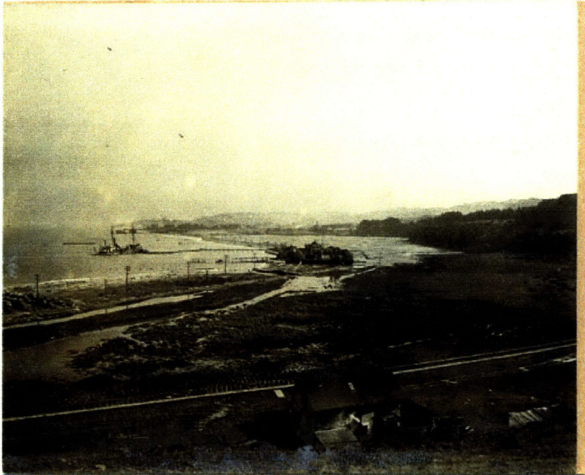
Filling of the wetlands begins. Note offshore barge used to pump sand and. Also, note remaining marshland in foreground. (SFPL)
