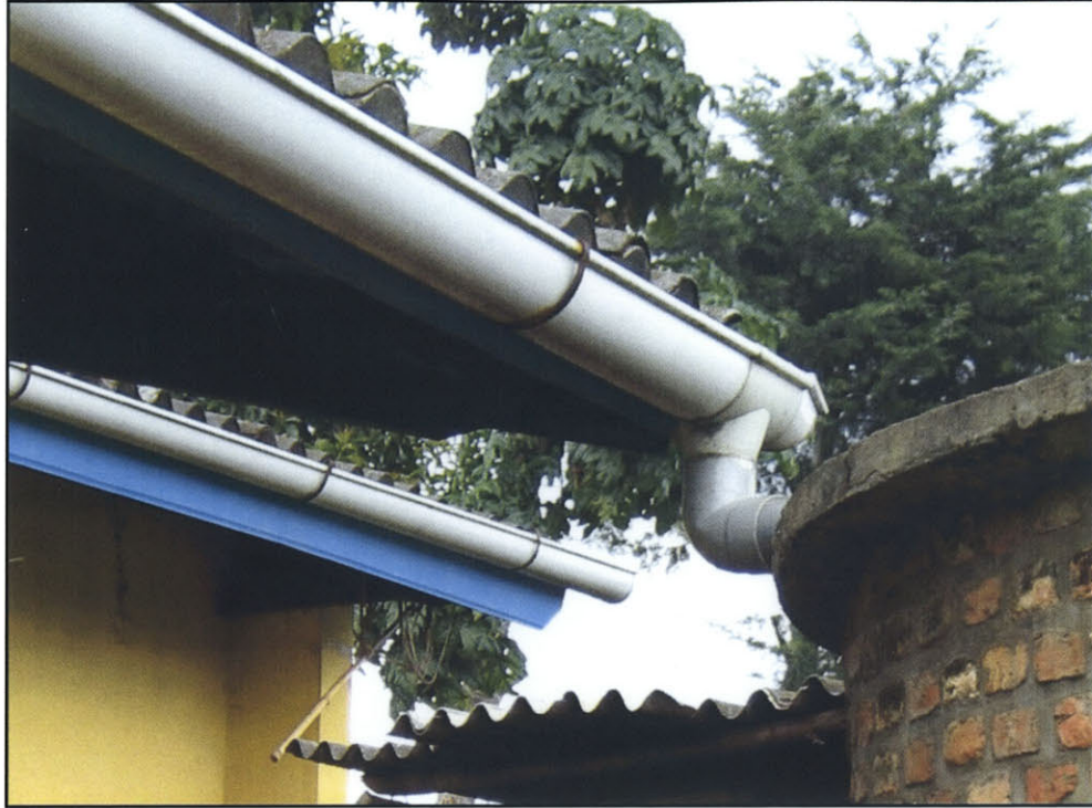
Figure 53: PVC semicircular gutters in Bisate Village (Picture by Author)
