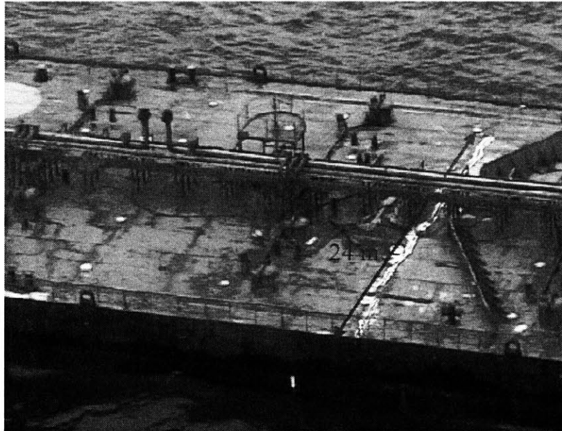
Figure 3-1: Macro-crack of 24 m in length on the weather deck of the tanker Castor [113] [courtesy of IMO]
