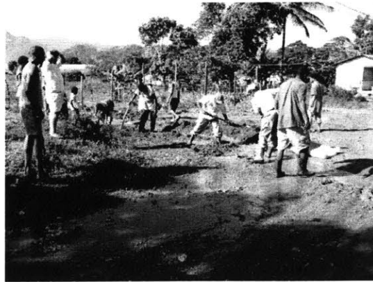
Figure 4-6: People had brought their own shovels and pickaxes, but there were more people than tools or space to work.
