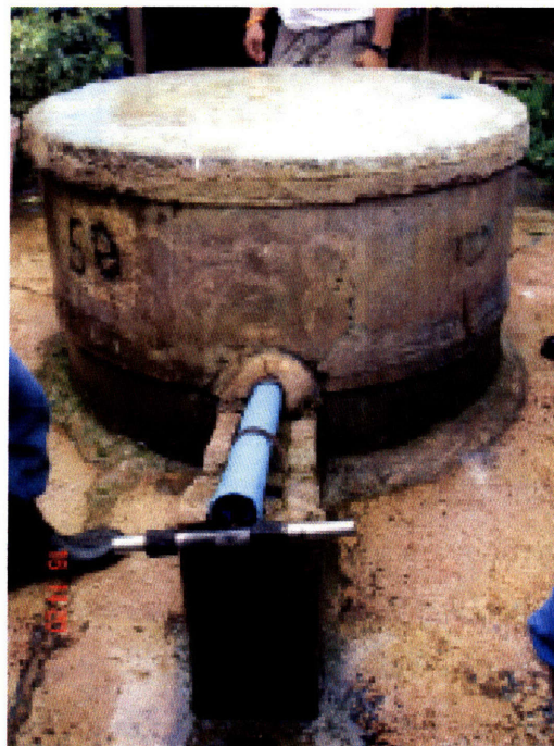
Figure 1-5: Typical rope-pump well (Lantagne, 2007)
