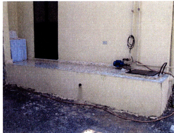
Figure 10. Underground cement cistern.
