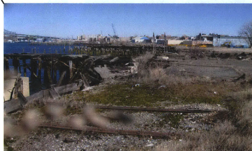
Dilapidated piers, concrete foundations, and marine railways, largely on the DPA portion of the site.
