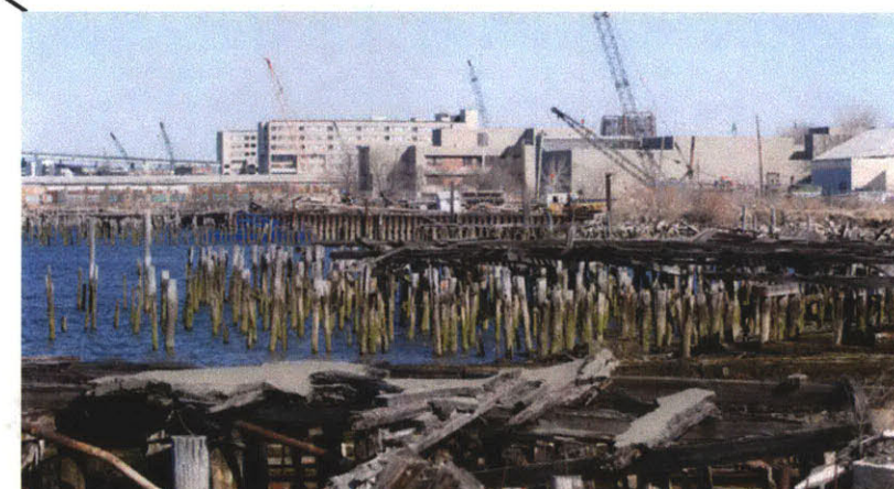
Dilapidated piers, along the sites watershed with building cranes in the distance.
