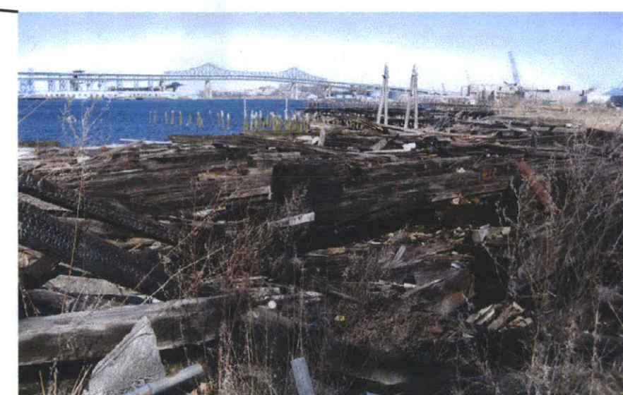
A decayed pile of timbers from historical wharves make up part of the ground plan of the DPA portion of the site.
