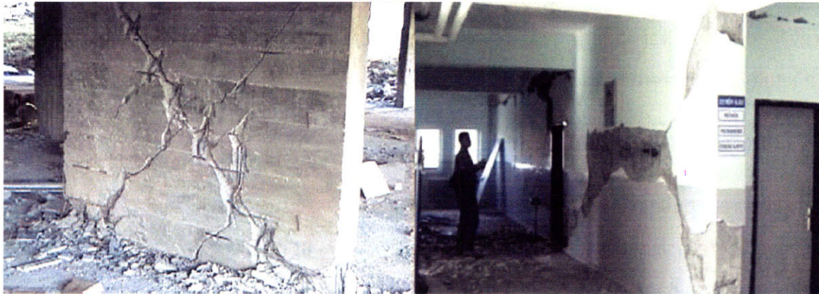
Figure 7: Shear failure of RC walls (Ireland et al. , 2006)
