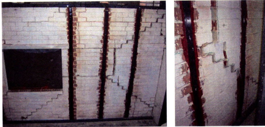
Figure 23: Damage to URM walls retrofit with vertical FRP strips (Willis et al. , 2009)
