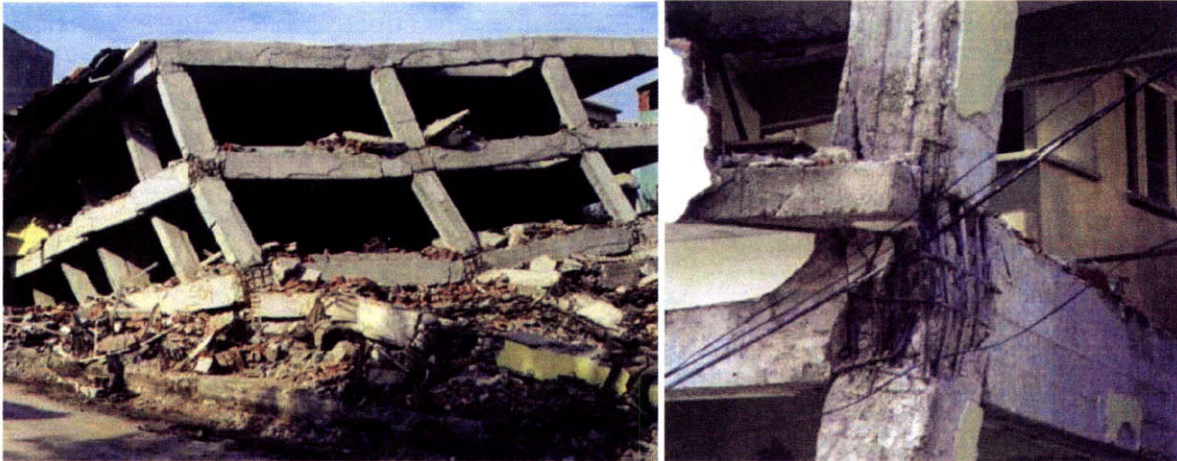
Figure 6: beam-column joint failure in typical reinforced concrete frames (Saaticioglu et al. , 2001)
