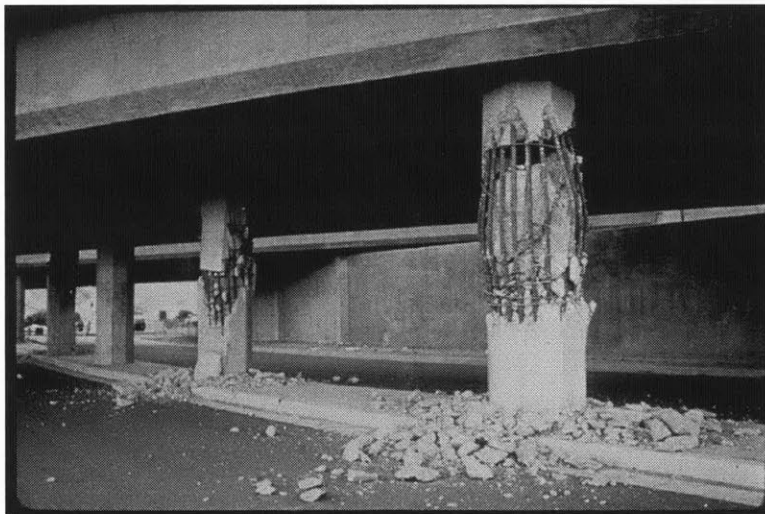
Figure 14 : Failure of several columns, Foothills Freeway overpass. Spalling due to an earthquake
