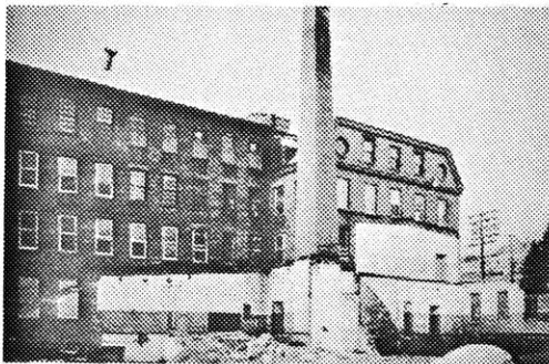
Entry facade showing cementitious paint after demolition of 2 additions, and chimney stack before demolition.
