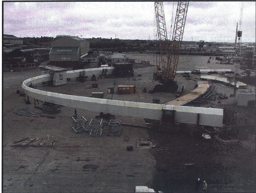
Figure 4.2 – Assembly of the arch and deck at the staging ground. Note the three deck sections to the right of the image. (Courtesy of Paul Kassabian, Waston Steel)
