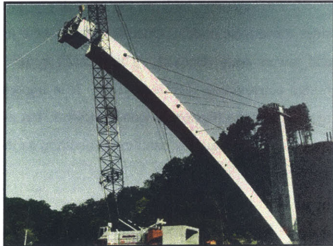
Figure 2.6 – The first segmentally constructed concrete arch bridge in the U.S., Natchez Trace Parkway, Franklin Tennessee. (Courtesy of U.S. Department of Transportation)
