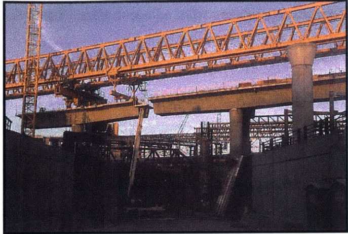
Figure 2.9 – Launch Gantry at Boston’s Central Artery Tunnel Project (Courtesy of the Massachusetts Turnpike Authority)
