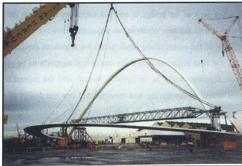
Figure 4.5 – Temporary shoring tower repositioned for lifting of assembled bridge. (Courtesy of the Gateshead Metropolitan Borough Council)
