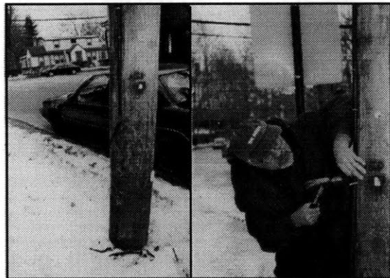
Repair of the plastic conduit representing the door post by an eruv checker
