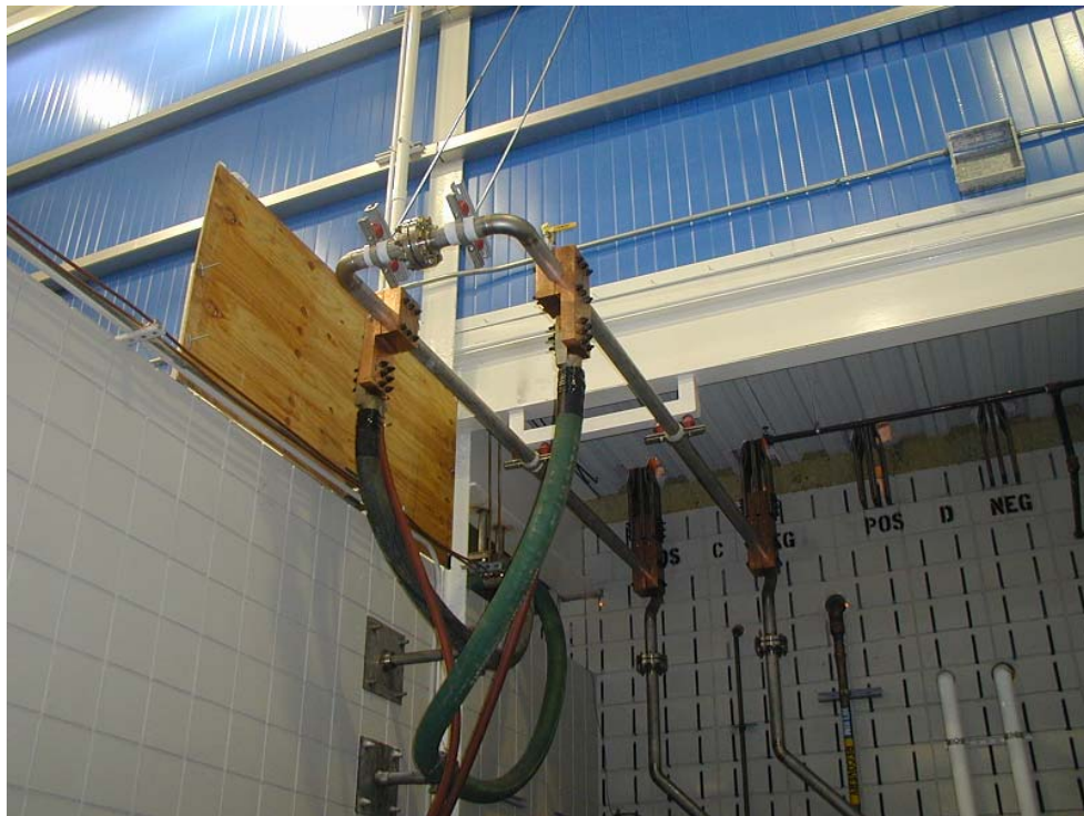
Fig. 27 20 kA cables and water cooled resistor to improve the stability of the voltage power supply.
