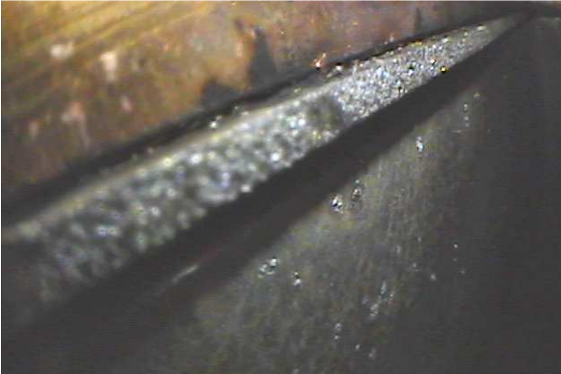
Figure 2-6: Arc damage at the RWA/FWA interface due to misalignment of the gasket. The copper shaded region in the upper left is the FWA, and the silver region in the lower right is the RWA. The gasket runs diagonally through the picture. This view is from the bottom of column 23, row C looking up along the broad wall of the waveguide. Splatter from melting of the gasket can be seen on the RWA.
