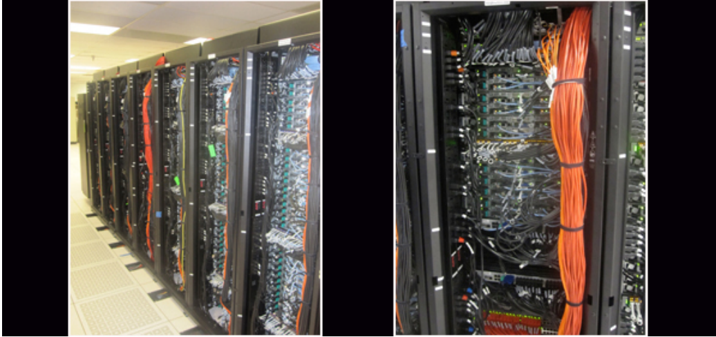
Figure 1.1: Example of electrical wiring in the supercomputer at Goddard in the year 2014. From [ http://geeked.gsfc.nasa.gov/?p=3601 ].
