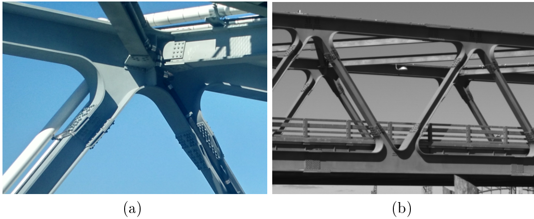
Figure 7-22: Pictures of the special connections on the bridge with a monolithic joint and the gusset plates moved onto the elements with pictures from the (a) bridge interior showing diagonal supports between the trusses and (b) bridge exterior
