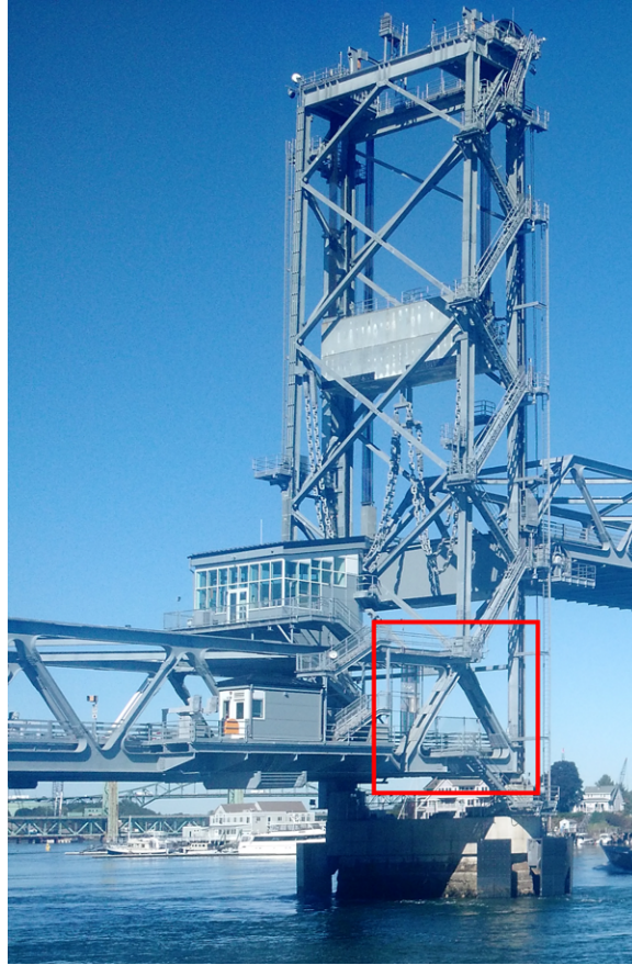
Figure 7-23: Picture of the south tower and fixed truss with the truss-tower connection outlined in red showing gusset plates tying the two together
