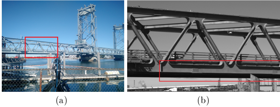
Figure 7-4: (a) Picture showing the view from the camera measurement location with the video area outlined in red and (b) screenshot of the recorded video with a region of interest for the bottom chord of the bridge outlined in red
