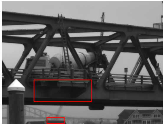
Figure 7-16: Screenshot from the start of the 10:21:03 am video showing a concrete mixer truck and regions of interest on the bottom chord and an object in the background
