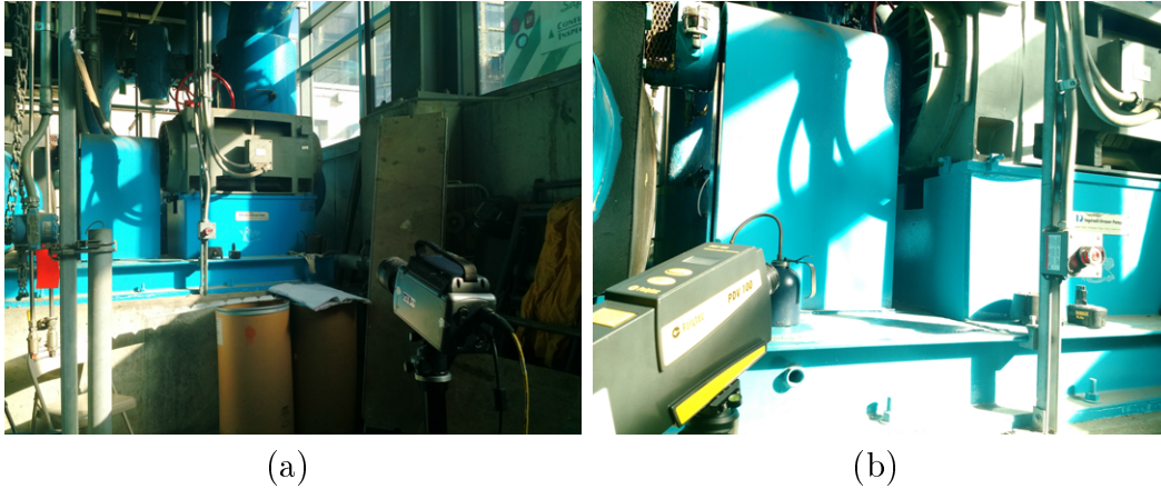
Figure 6-1: Measurement setup for the motor that drives a chilled water pump showing (a) the camera location relative to the pump and (b) the laser vibrometer positioning
