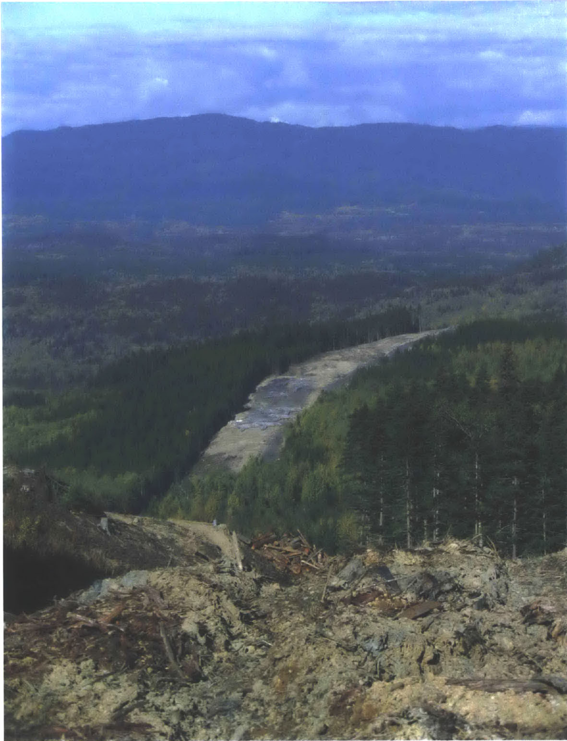
FIG 4.6. A 100 m wide right-of-way through Gitanyow territory cleared for the Northwest Transmission Line. The preponderance of post-clear cut second-growth forest (the shorter, multi-colored tree stands, versus the darker areas along the far ridge) throughout the region becomes visible immediately when seen from above.
