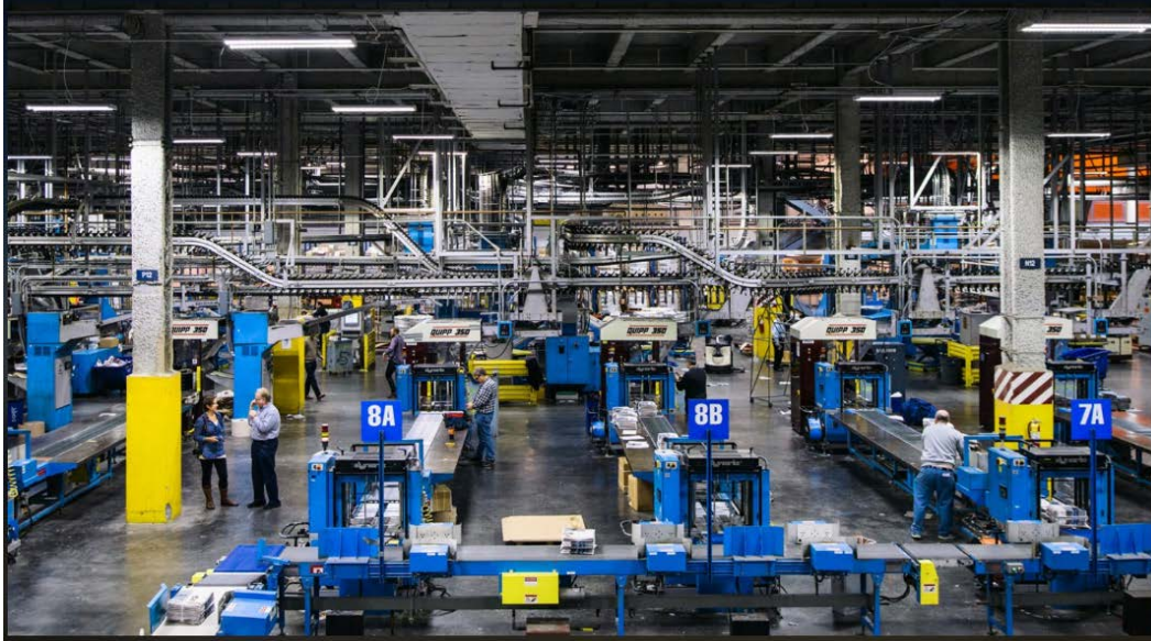
Fig 1: Partial view of one of the floors of a NY Times printing facility (1 NY Times Plz, Flushing, NY 11354)
