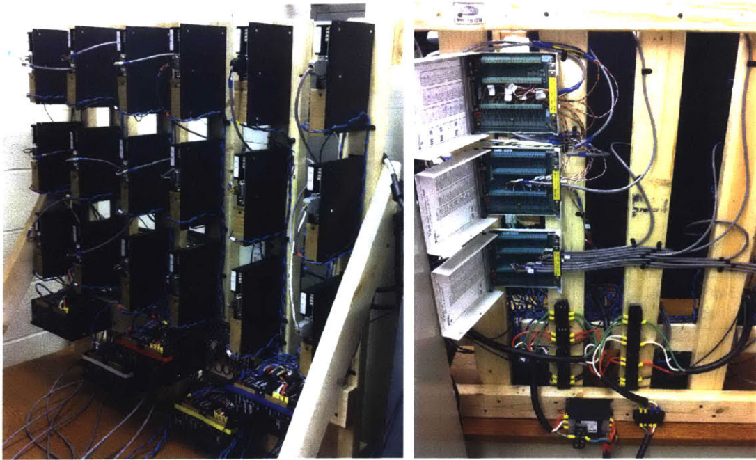
Figure 5-20: Customized rack for 5 power supplies and 18 power amplifiers: front view (left) and rear view (right).
