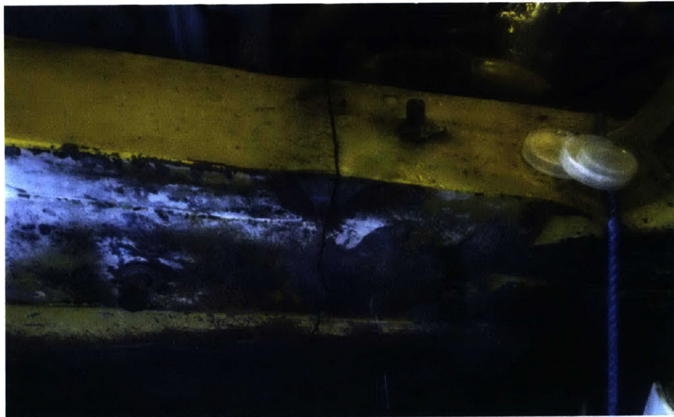
FIGURE 1: VIEW OF CRACK ORIGINATING FROM LARGE GROOVE WELD DEFECT
