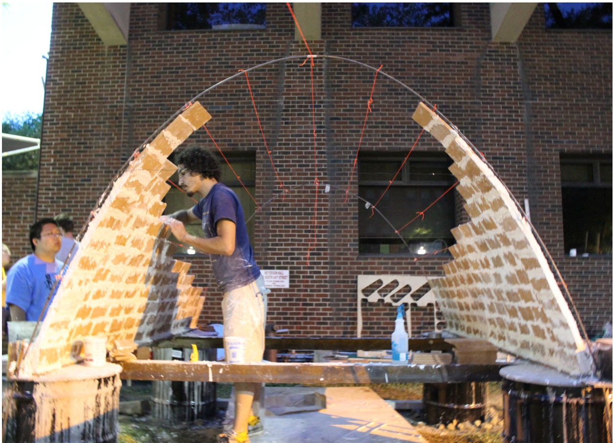
Fig. 1.8. "Cowboy Construction" [not to be attempted except under strict supervision]. Constructing an extruded arch (barrel vault) without support in Philadelphia. From [Dessi-Olive, 2014].
