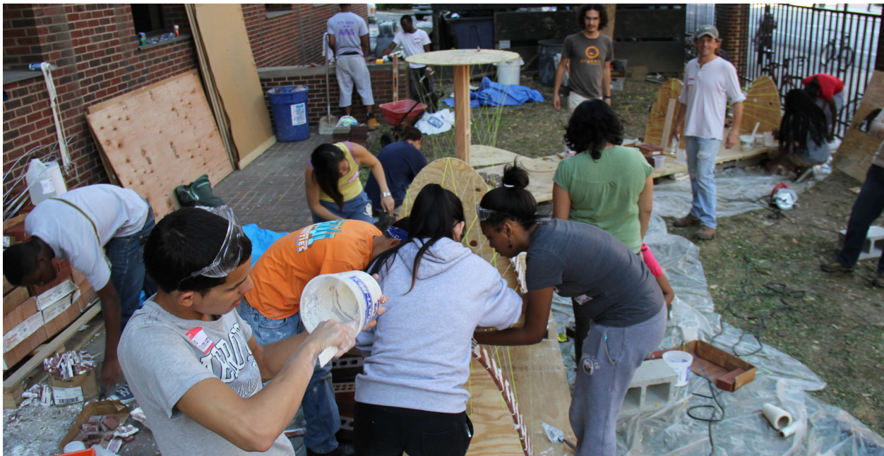
Fig. 0.5. Tile Vault Construction Workshop with Professor Franca Trubiano, PennDesign and students from the Charter High school of Architecture and Design (CHAD) in Philadelphia. Fall, 2013.
