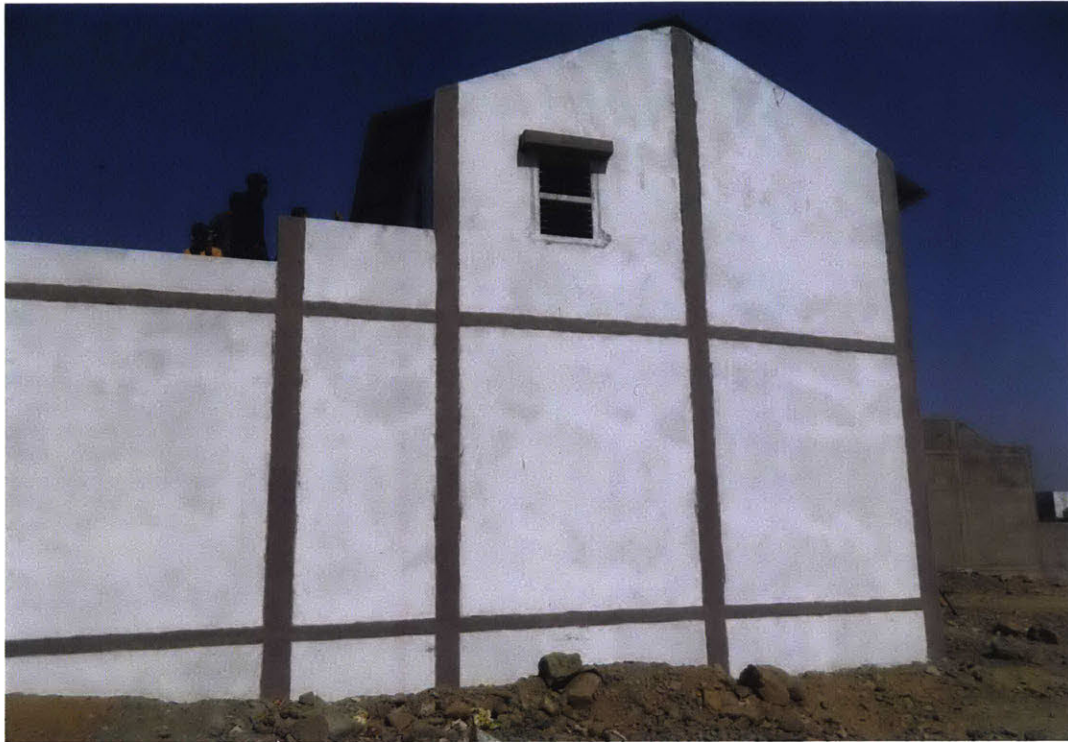
Exterior of Housing for All Home with a Double Layer Tin Roof and Wood Ceiling
