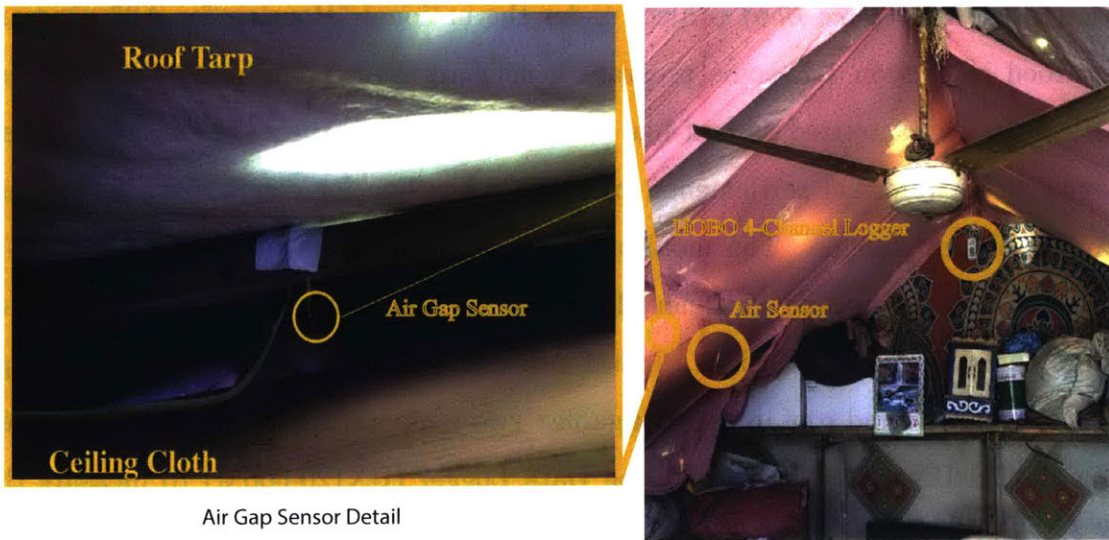
Figure 3-2: Interior Ambient Air and Air Gap Sensor Placement in Informal Home
