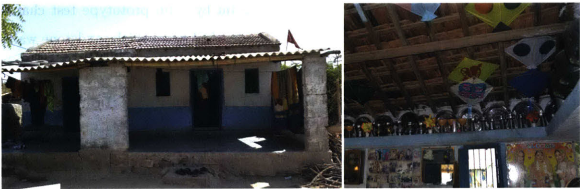
Figure 1-8: A Stand-Alone Two-Room Dwelling with 15cm Thick Uninsulated CMU Walls and a Single-Layer Mangalore Pattern Tile Roof (Gradillas, 2015)
