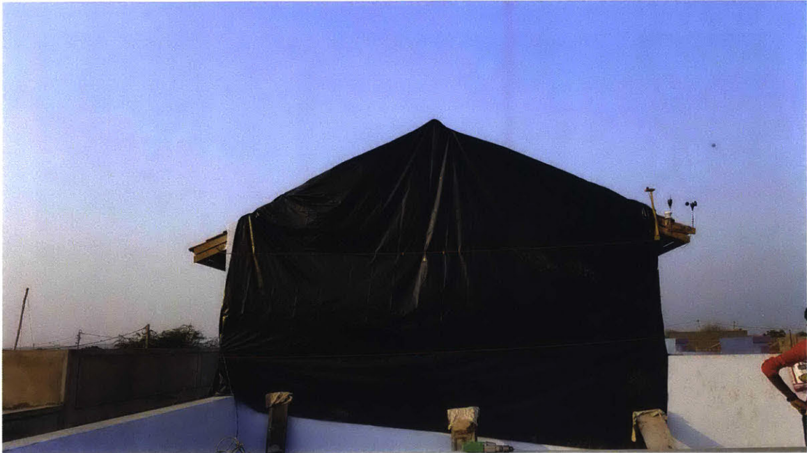
Figure 5-16: Black Tarp Covering the South Wall of a Monitored Housing for All Home with a Multi-Layer Mangalore Tile and Mud Roll Insulated Roof
