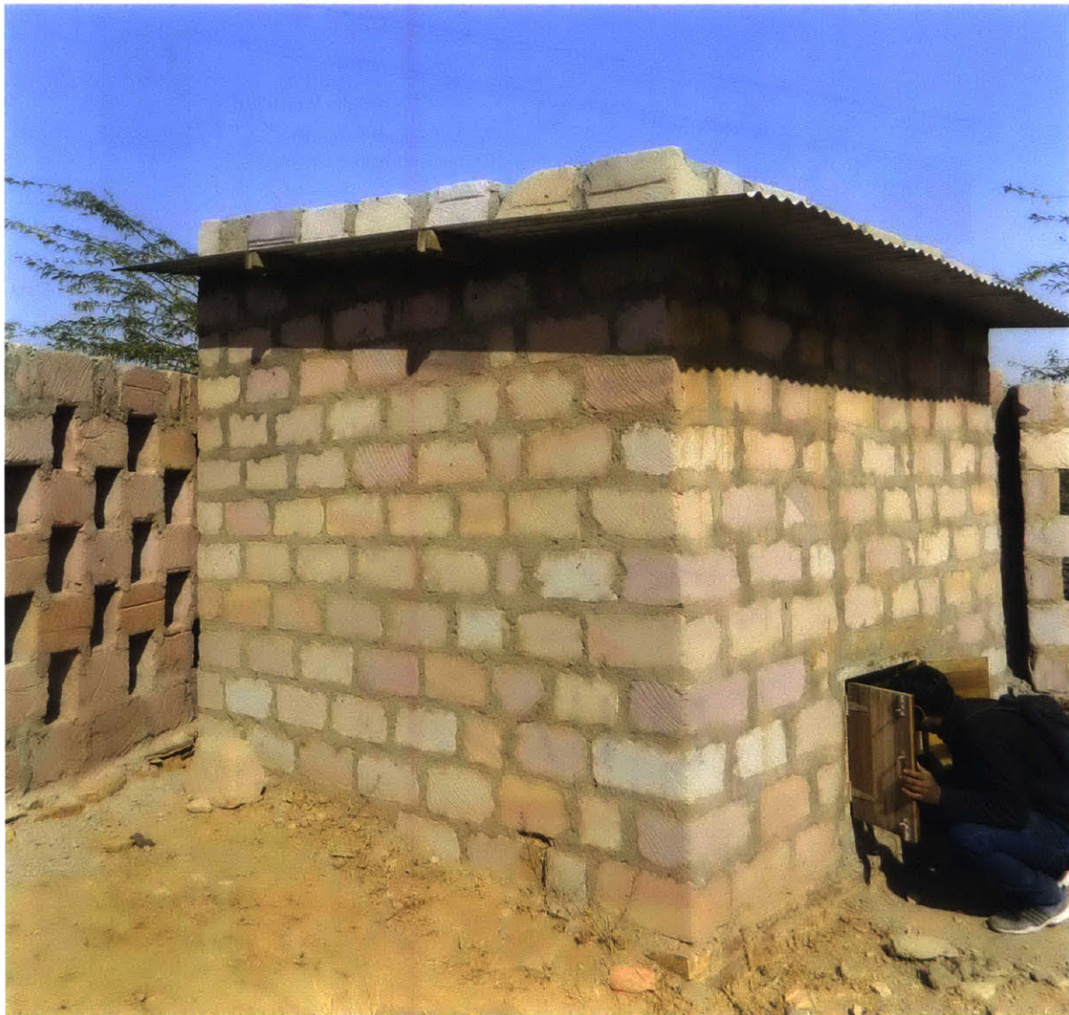
Figure 7-4: Exterior View of Test Chamber with Single Layer Roof (Photo Courtesy of John Kongoletos)
