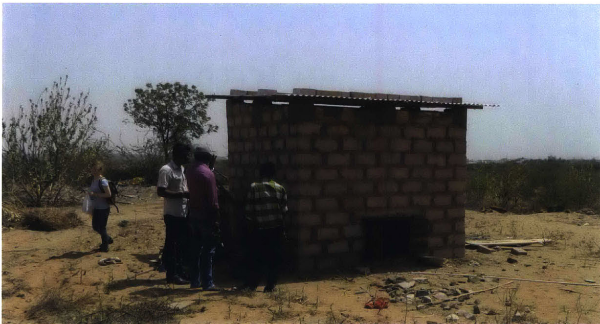
Figure 7-6: Exterior View of Test Chamber with Double Layer Roof (Photo Courtesy of John Kongoletos)
