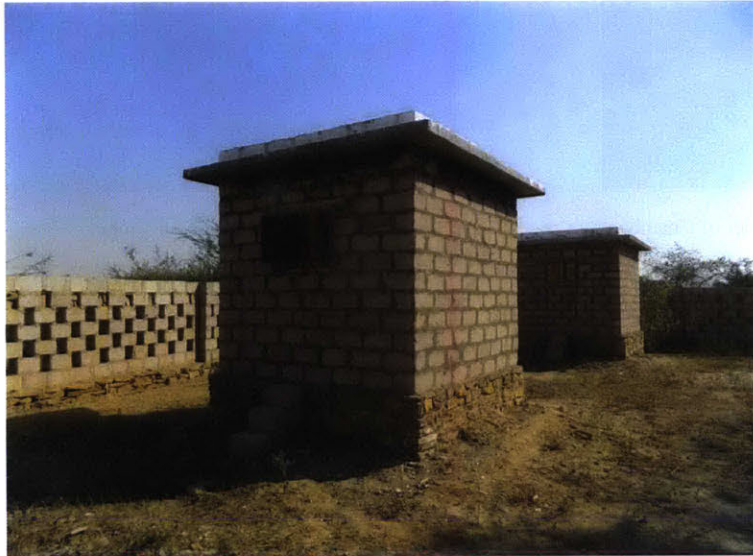
2.4m Cubed Test Chambers with 23cm Thick Sandstone Walls and Ventilation Windows
