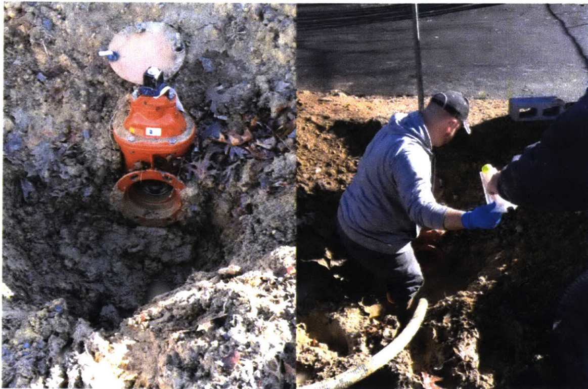
Figure 2-24: Picture of the Tee junction for robot entrance (left) and PSA Technician Steven Jenkins manually placed the robot in this Tee
