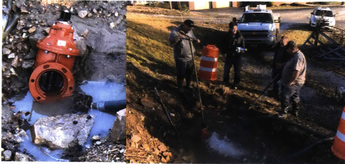
Figure 2-25: Left: Picture of the Tee junction for robot exit. Right: Picture of shutting the Tee junction off after the robot was retrieved. The persons in the picture from left to right are Steven Jenkins(PSA), You Wu(MIT, holding the retrieved robot), Alan Harrison(PSA) and Shane Clark(PSA).
