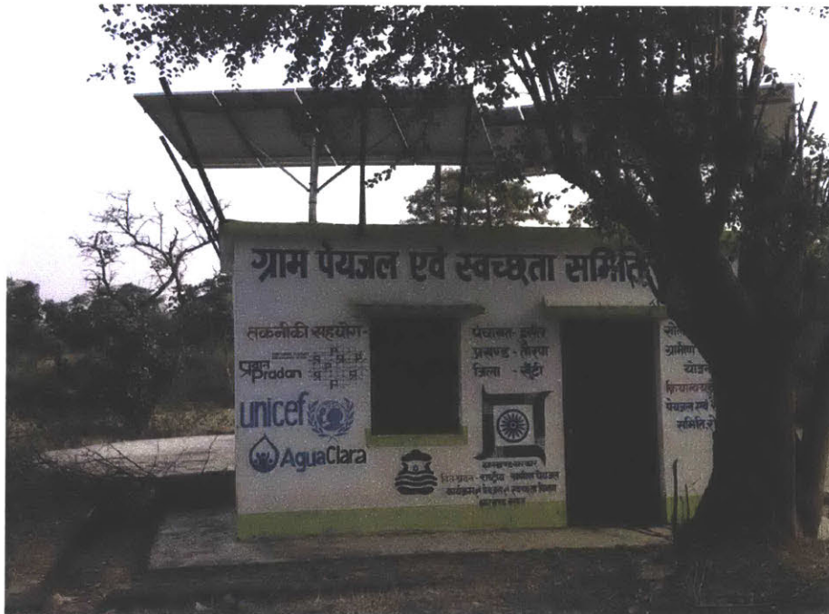
Solar Pump for Water Tower in Rohne, Jharkhand
