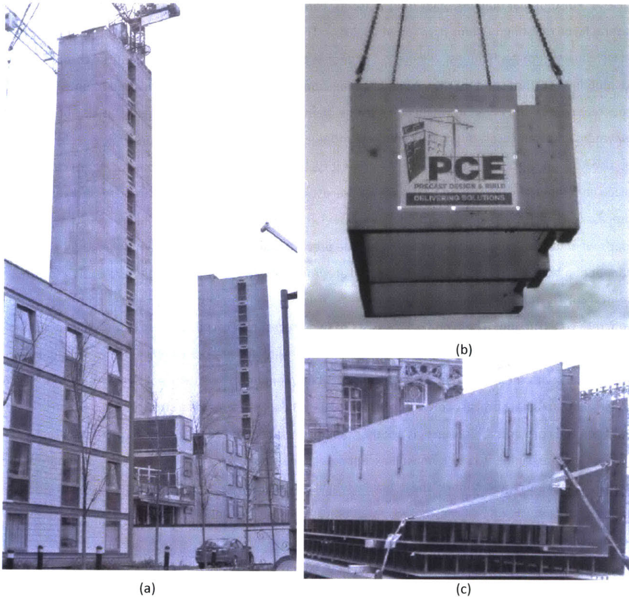
FIGURE 2.3 - MODULAR CORE SYSTEMS. (A) PARAGON UK, CASE IN PLACE (B) PRE-CAST (C) COREFAST SYSTEM (CALEDONIAN MODULAR, MAY 2018)
