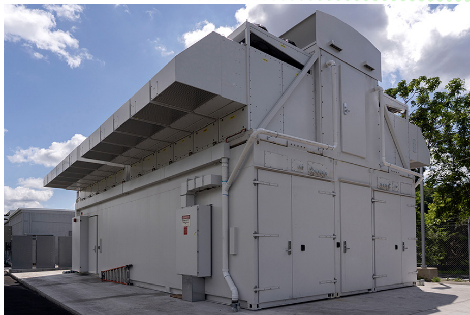
TX-GAIA is housed inside of a new EcoPOD deployable data center, manufactured by Hewlett Packard Enterprises, at the site of the Lincoln Laboratory Supercomputing Center in Holyoke, Massachusetts.
