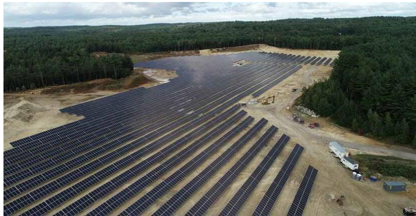
Figure 22 – The Happy Hollow Solar Farm built on a former gravel pit 45
