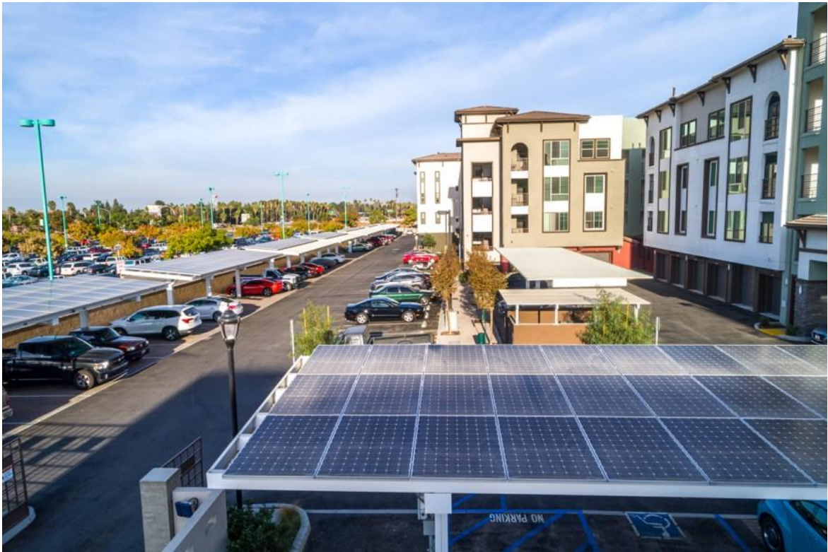
Figure 20 – Solar Carport in Southern California 40
