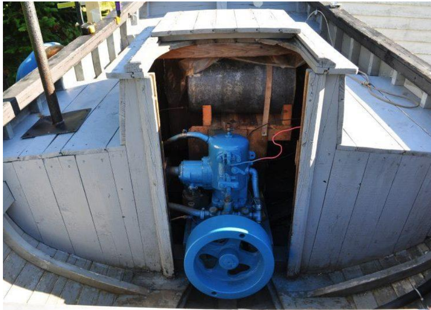
Figure 1-1: Atlantic Marine engine installed in the back of a boat [1]
