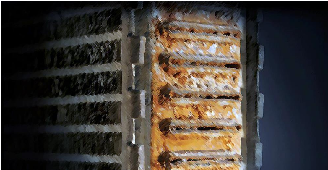
Corrosive effects of chlorides on data center equipment, Image: Artistic Rendering by Author
