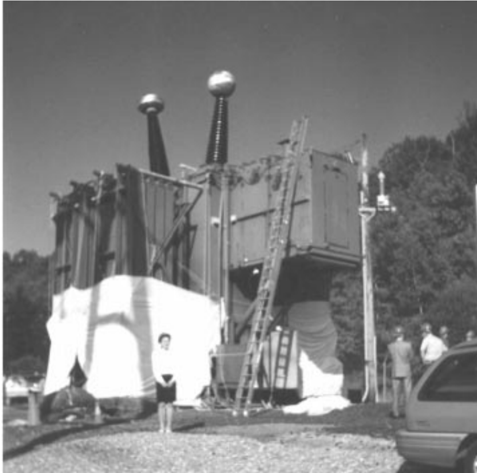
Figure 1.2: The author in front of one phase of the Ramapo Substation Westinghouse 500/345kV, 333 MVA auto transformer.
