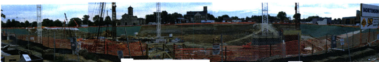
fig. 10. Panorama of construction site for the New Memphis Arena, an area just south of Beale Street
