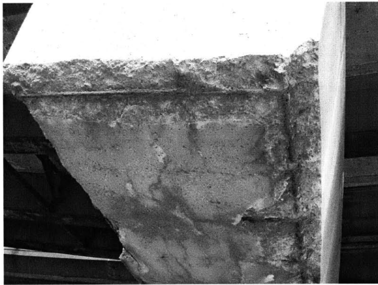
Figure 6. Extensive Damage Due to Reinforcement Corrosion
