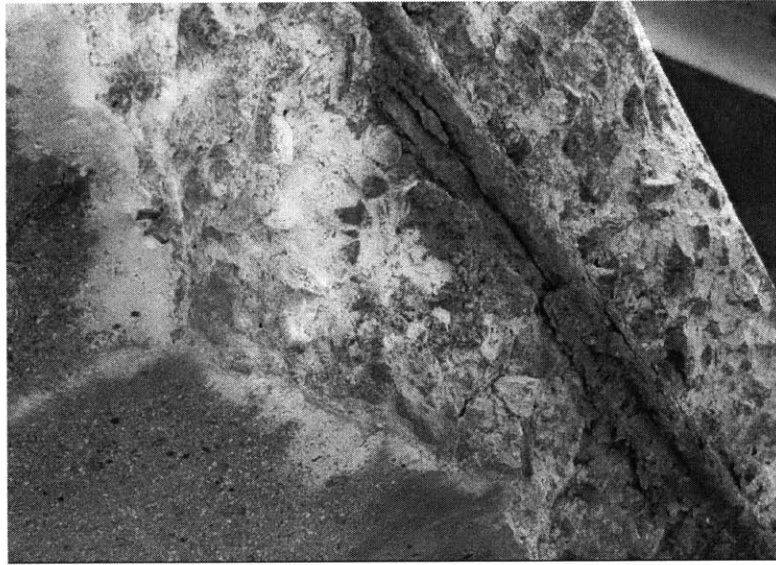
Figure 5. Spalling Due to Reinforcement Corrosion
