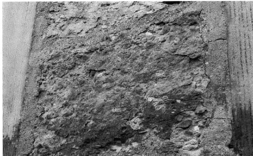
Figure 3. Concrete Damage Due to a Corrosive Environment
