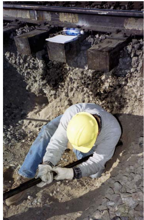
Figure 5.20: Hand installation of the probe in the augered hole using a rod.
