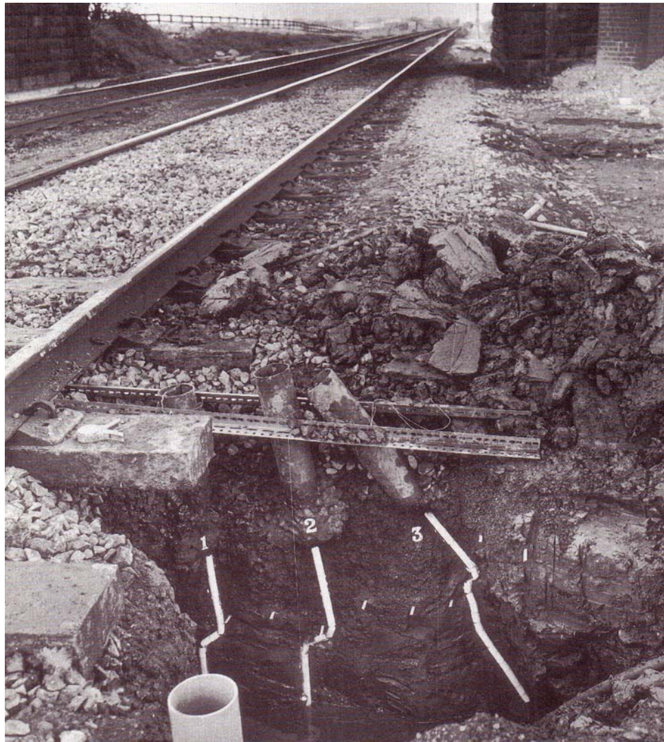
Figure 2.3: Distorted columns indicating progressive shear failure. (SELIG & WATERS 1994)
