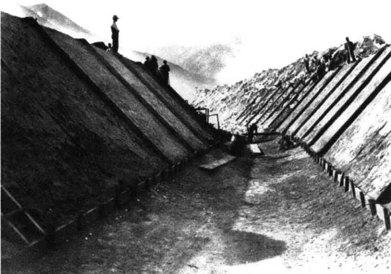
Formwork being installed for the open concrete-lined channel. Photo from the LADWP archives.
