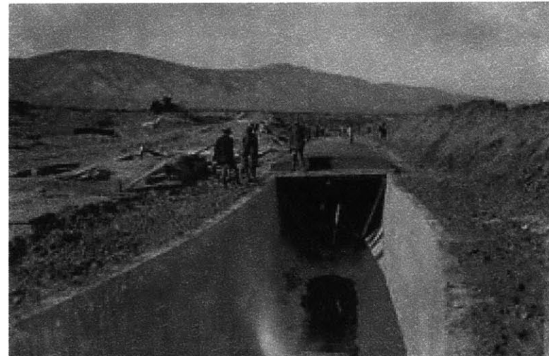
The box-shaped concrete form, called a conduit, continued down to Los Angeles interspersed with tunnels and siphons. Photo from the LADWP archives.
