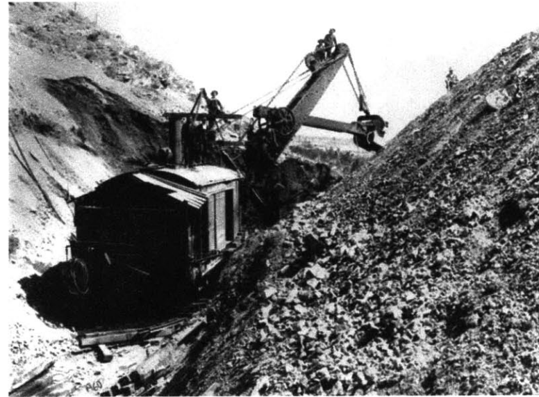
The earth was excavated with a dipper dredge then discharged away from the channel. Photo from the LADWP archives.
