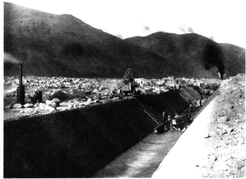
Construction of the LAA open concrete-lined channel east of the Alabama Hills. Photo from LADWP archives.
