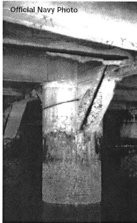
Figure 9: Navy Marine Structure with Extensive Corrosion Damage
