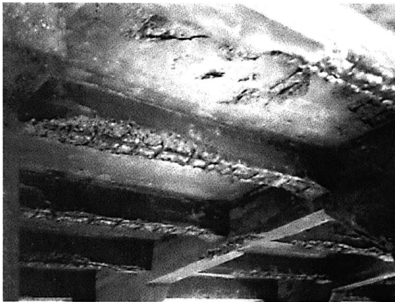
Figure 8: Extensive Black Steel Rebar Corrosion on Parking Garage Ceiling
