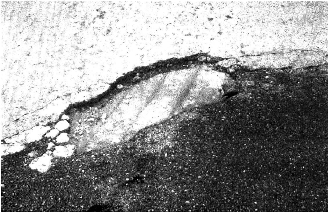
Figure 2: Concrete Spalling with Exposed Reinforcement
