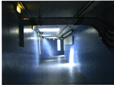
Figure 3-b6, left: The computer room
