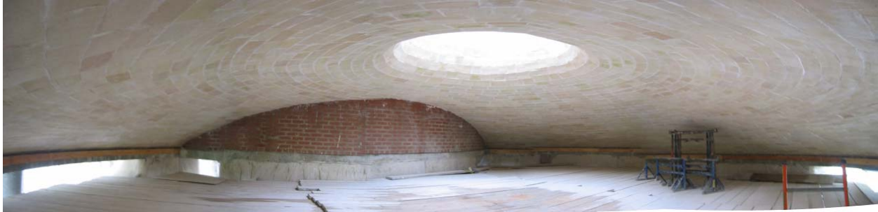
Figure 5.12. The interior of the lower dome of the Pines Calyx near the end of its construction (photograph courtesy of Michael Ramage)
