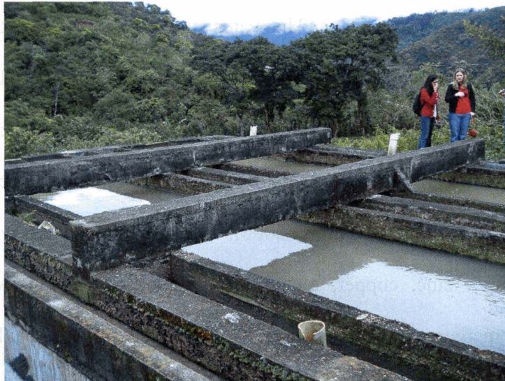
Figure 4.5: Wastewater treatment facility, Municipality of Las Vegas
