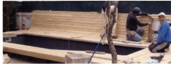
Traditional woodworking fabrication of a curved surface Valenzuela's House, Santiago, Chile 2004 Picture taken by the author, 2004.
