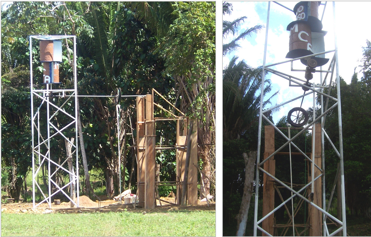
Figure 1: Two views of the wind-powered water pumping system installed on the property of the Nuevo Paraiso Enterprise in Guadalupe Carney, Honduras.
