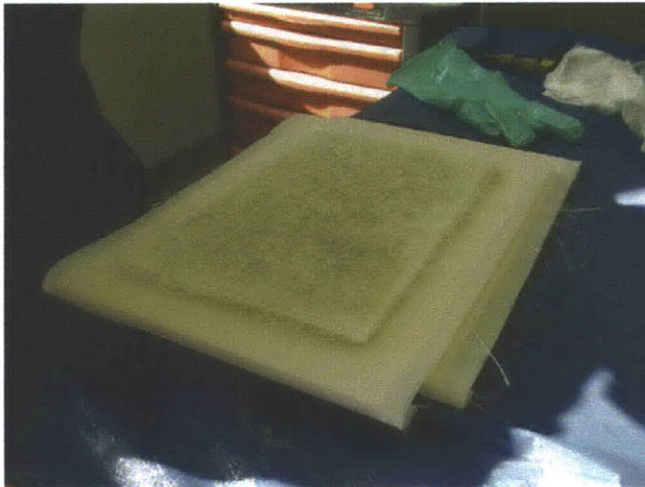
Figure 2.25 Ten layers of fiberglass mats wetted through epoxy on the bottom mold
