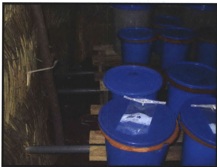
Figure 4-28: Pipes Carrying Water From 24 Filters Through Grass Mat Walls
