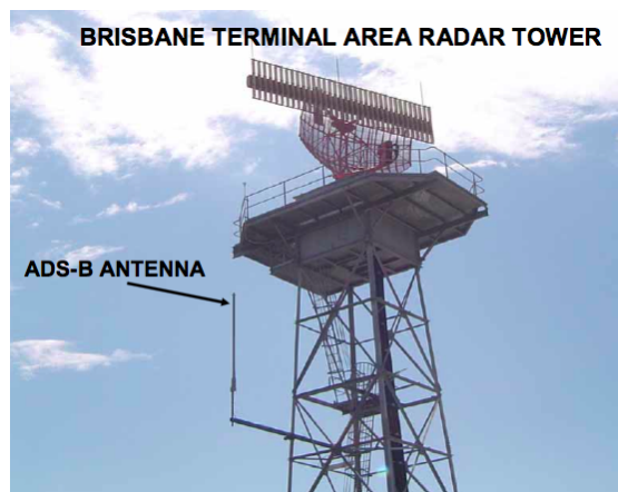
Figure 8: Temporary Installation of an ADS-B Antenna on a Terminal Area RADAR Tower in Brisbane, Australia (credit: Greg Dunstone)
