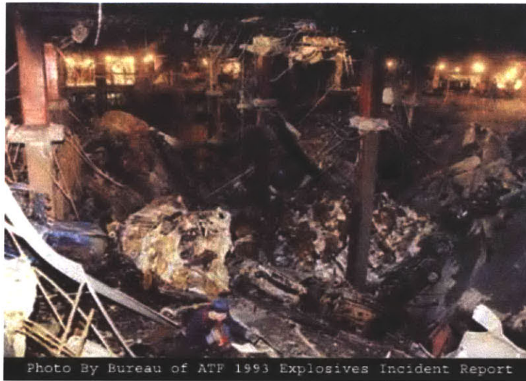
Figure 1.1 View of damage from 1993 World Trade Center bombing (Source: geopolicraticus.wordpress.com )
