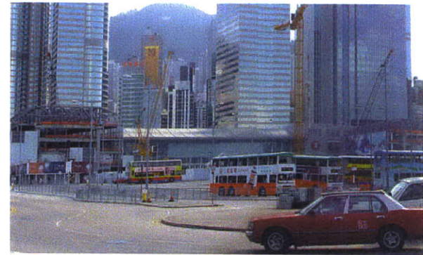
Photo of the New Hong Kong Station Still Under Construction Awaiting the Completion of its Hotel Wing.
